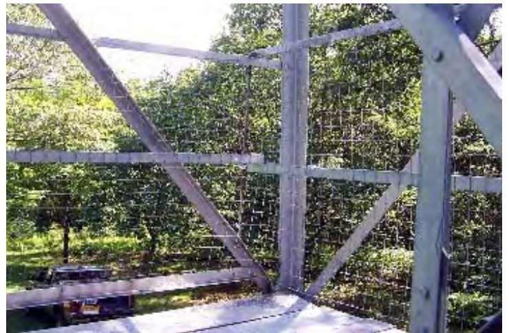
Mid-rail and wire safety meshing on a landing.
